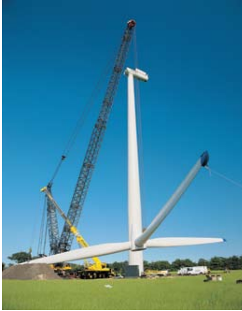
Large wind farms can need up to 300 workers on site during construction. Credit: BONUS Energy A.S.
